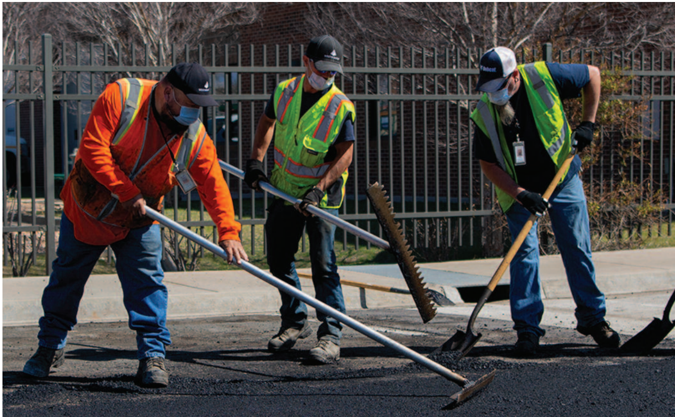
Public Works and Utilities Department employees wear masks and practice social distancing while repaving the Municipal Service Center. L to R: Crewleader Mike Cabral, Street Maintenance Worker II David Mortier, and Equipment Operator I Gary Aldrich.
