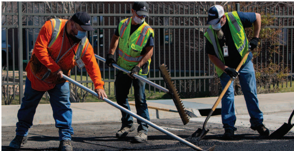
Public Works and Utilities Department employees wear masks and practice social distancing while repaving the Municipal Service Center. L to R: Crewleader Mike Cabral, Street Maintenance Worker II David Mortier, and Equipment Operator I Gary Aldrich.
